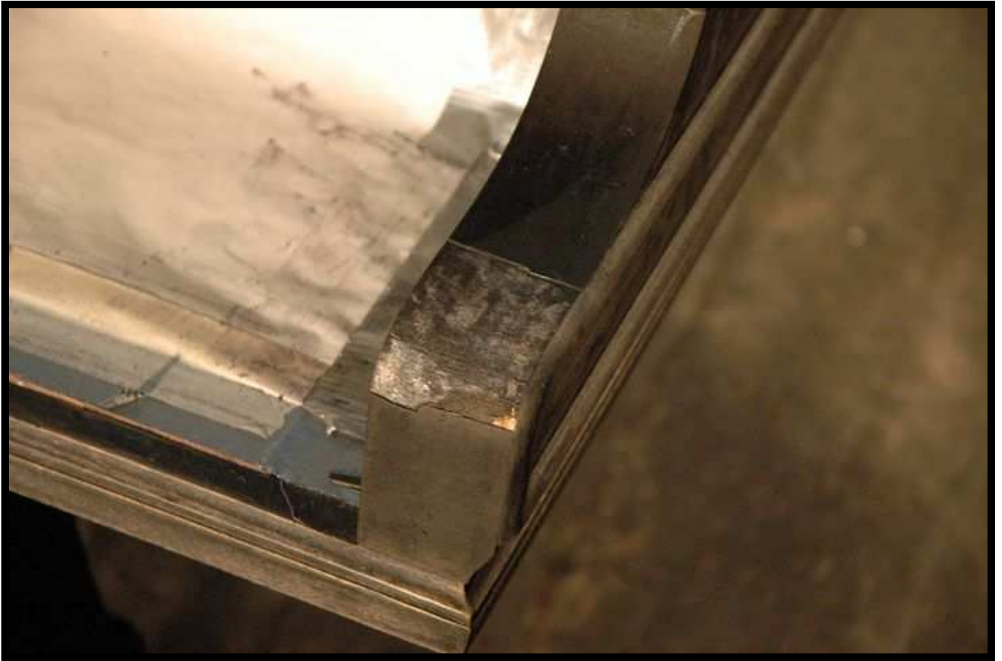
Detail of some damage to be repaired. prior to application of the primer coats.
