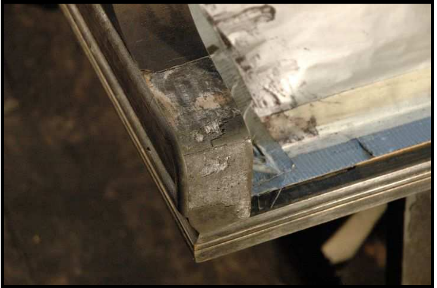
Detail of more damage to be repaired, prior to application of the primer coats.
