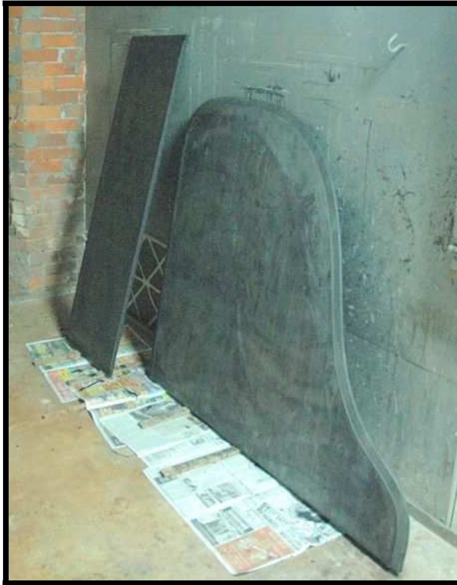
Top sections after stripping. Next step is rinsing with a special solvent to remove all residue, prior to refinishing with the same steps shown for the piano casing.
